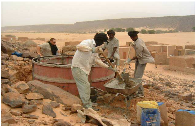
Figure 3. Water Project at Lemraiveg, Adrar Region, Mauritania
