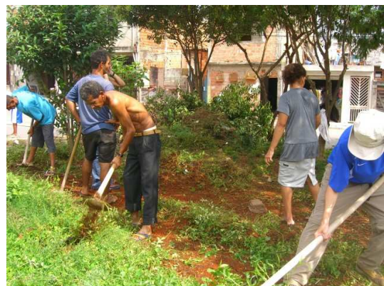
FIGURE 5 JARDIM CONCEIÇÃO: A SQUARE RENOVATION, WHERE THE STUDENTS WORKED TOGETHER WITH VOLUNTARY LOCAL PEOPLE.
